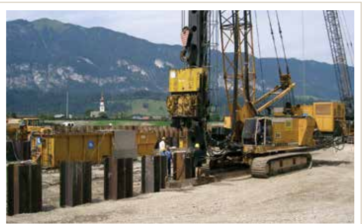
Fig. 11. Template with a single level and piling equipment guided on a fixed leader.
